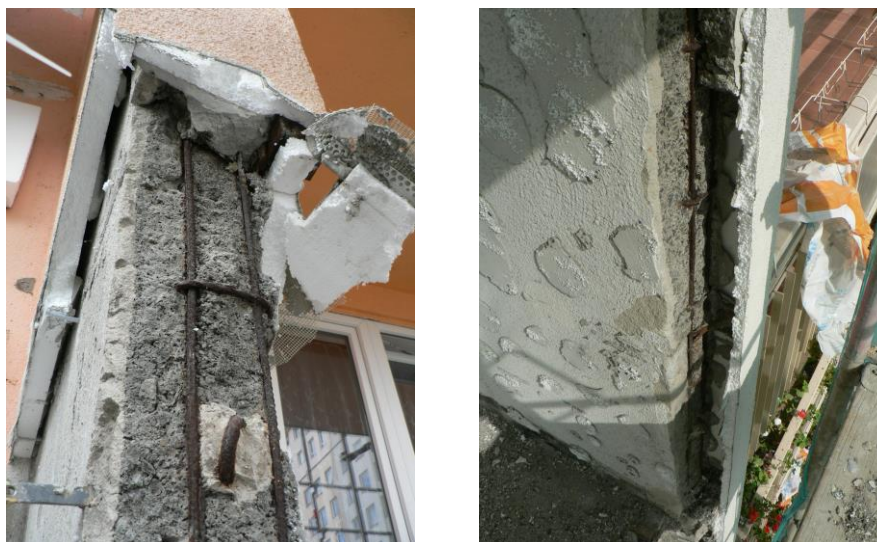
Figure 1. Failure of thermal insulation and concrete cover due to steel corrosion.
